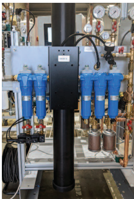
Medical air plant in SHJ's production facility in Chesham.
