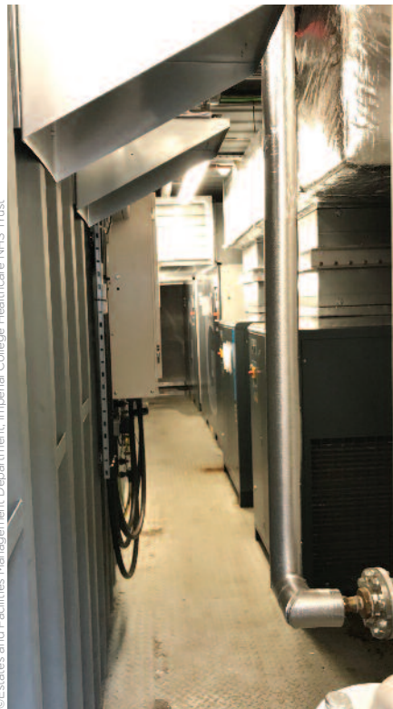
The compact plant layout in a standard high-roof shipping container.
