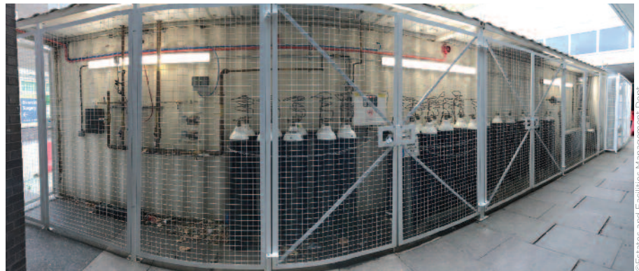
The oxygen concentrator connection and distribution manifold, and emergency standby manifold, arrangement.
