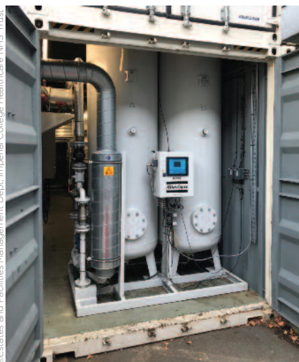
Oxygen generator vessels.
