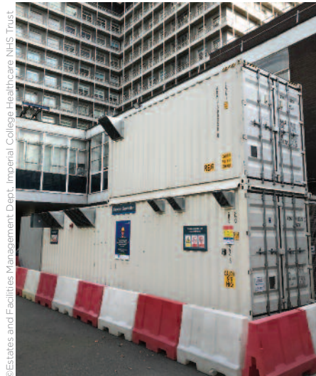
The container-sized plant room solution strategically located adjacent to the oxygen load.
