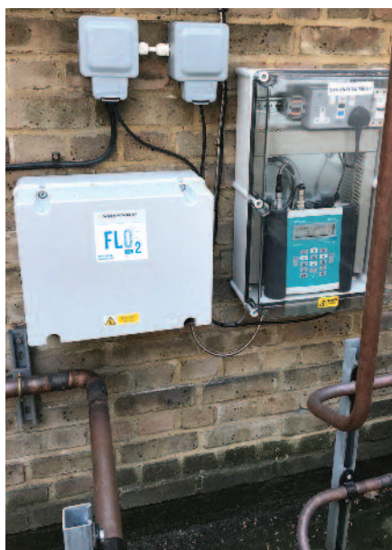
SHJ FLO 2 oxygen flow monitoring equipment installed at London's Royal Brompton Hospital.
