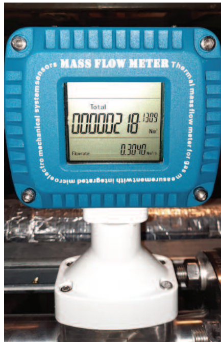
At Doncaster Royal Infirmary, SHJ recently installed nine FLO 2 boxes linked to integral flowmeters, enabling staff there to monitor nine 'take-offs'.
