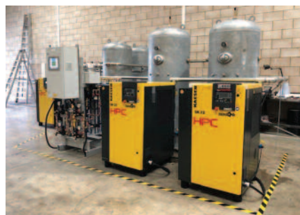
Many SHJ medical gas systems sold today will incorporate German-built Kaiser medical air compressors.
