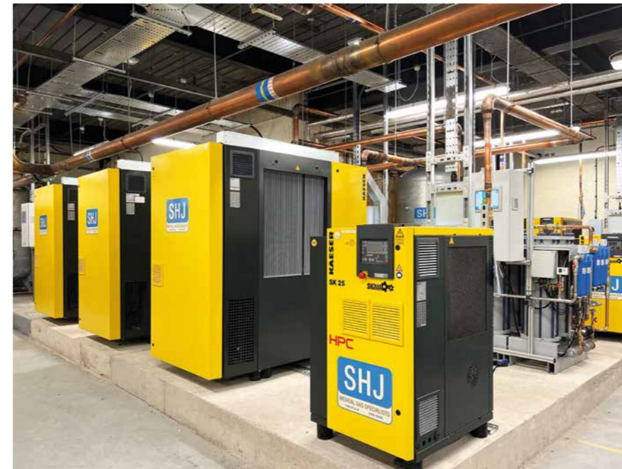
The RVI’s medical gas plant room.
