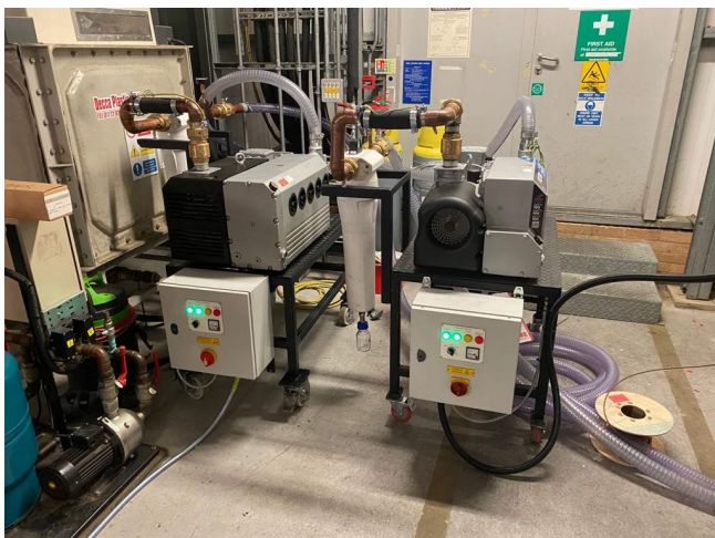
SHJ temporary plant, which keeps hospitals fully supplied with medical gases during installations.
